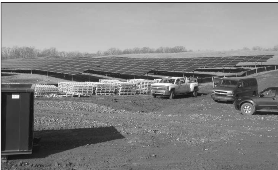
SOLAR FARM: Delaware River Solar, Inc. recently completed installation of New York State's largest community solar project on Baer Road in the hamlet of Callicoon. The 2.7 MW solar array has approximately 9,800 panels and will reportedly supply energy to more than 350 homes and businesses. It is located just outside the designated boundary of the Upper Delaware Scenic and Recreational River in the Town of Delaware. (UDC Photo by Pete Golod)
